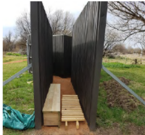
An incomplete mock trench in August 2017, with the first trial sections of fire step and duckboards, and the island traverse at its heart (Photo: Michael Maconachie).
